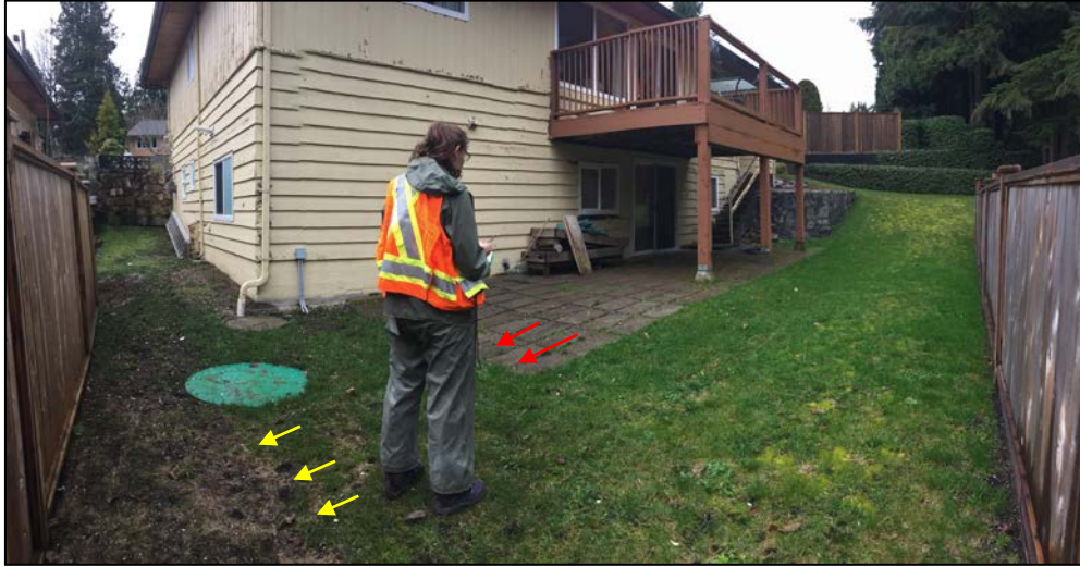
Photograph 8. 1582 Merlynn Crescent – Arrows show settlement of lawn near fence (yellow) and in patio stones (red).
