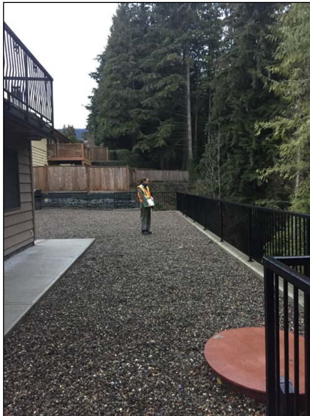
Photograph 2. 1576 Merlynn Crescent – Looking north across backyard with fence at the top of concrete retaining wall.
