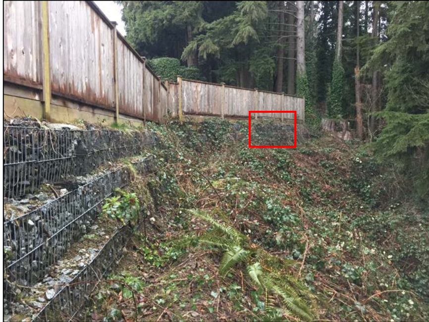
Photograph 6. 1582 Merlynn Crescent – Looking north at slope crest and GRS retaining wall. Red square showing location of close-up in Photograph 7.
