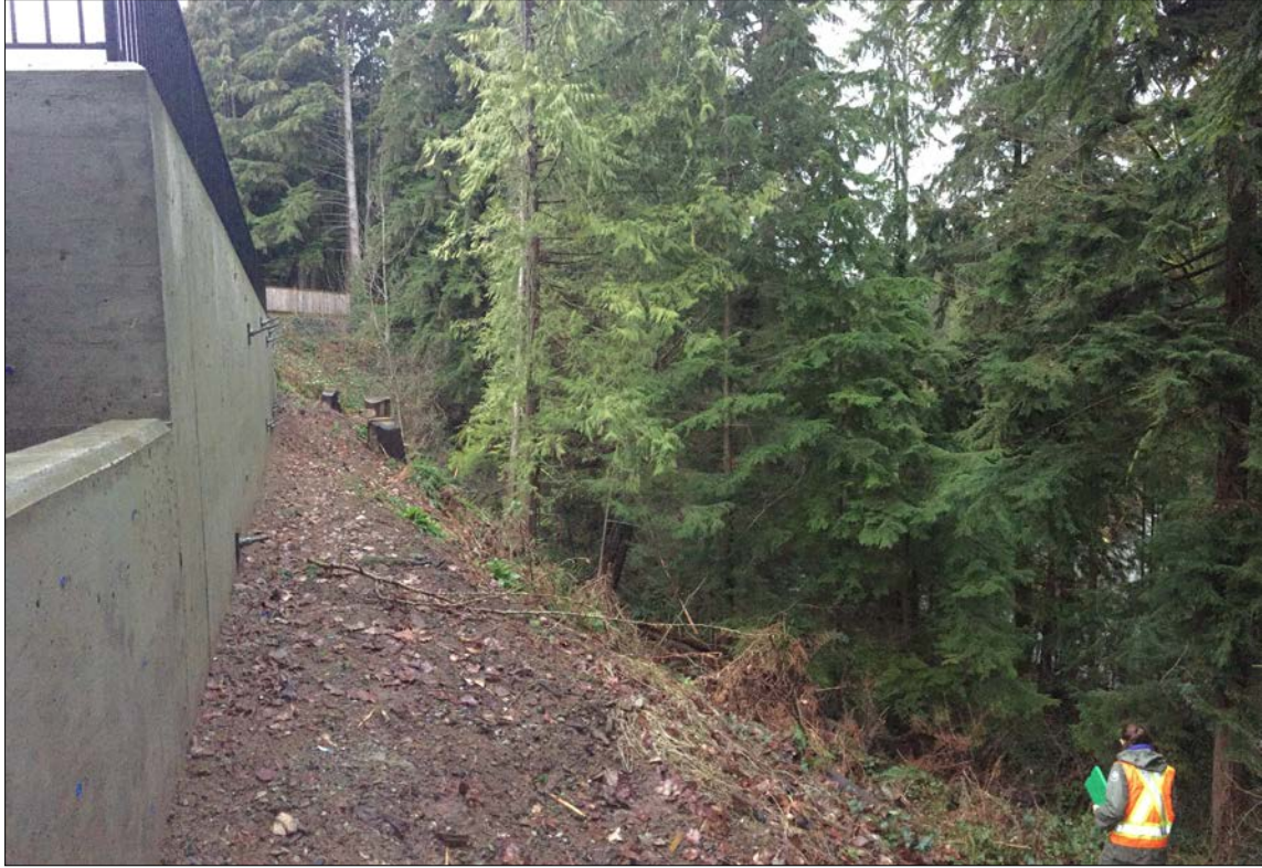
Photograph 3. 1576 Merlynn Crescent – Looking northeast at the escarpment slope below the concrete retaining wall.
