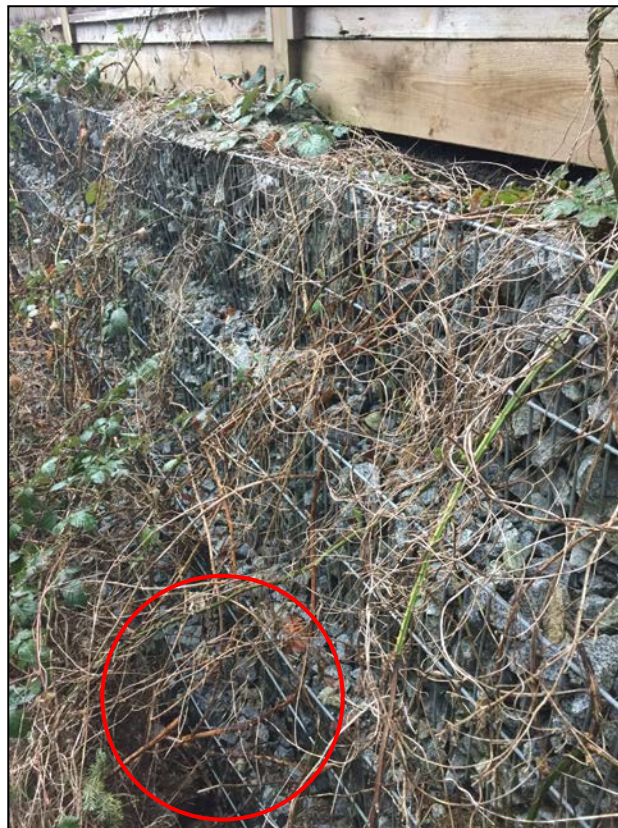
Photograph 7. 1582 Merlynn Crescent – Slight bulge (~ 10 cm) in lower row cage (red circle). This is interpreted to be the result of construction damage.
