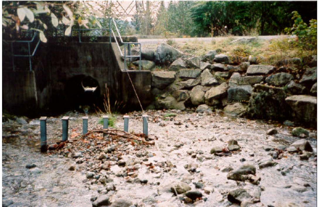
Photo F-7 Debris barrier at culvert inlet of Francis Creek, Indian River Drive. October 2001.
