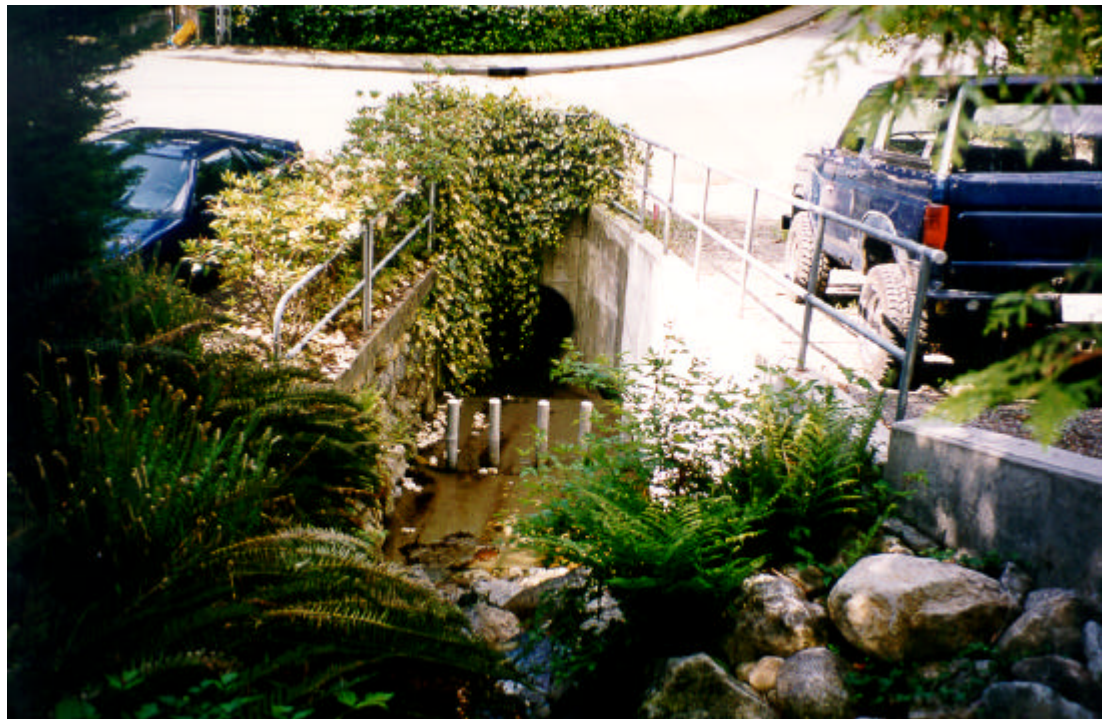
Photo MAR-2 Culvert inlet (1100 mm diameter) of Martin Creek at Panorama Drive. A small debris barrier is visible upstream of the culvert entrance. May 2002.
